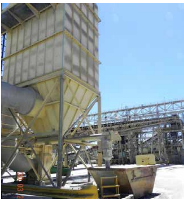
Figure 20: Fine crushing dust collection system
